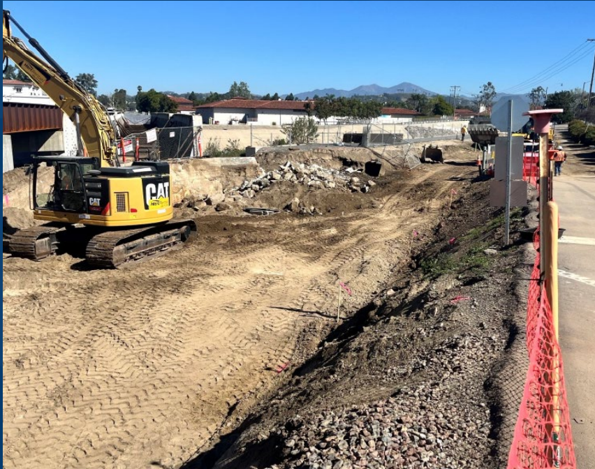
Abutment 4 demo and grading for temporary shoring – San Juan Creek Bridge Project
