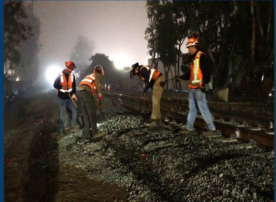
Dressing ballast on the north side of main track – San Juan Creek Bridge Project
